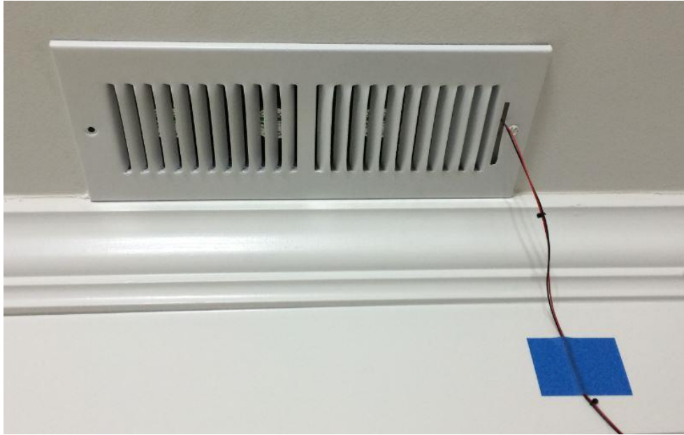
Figure 2-11 A register booster fan was attached to the duct register.
