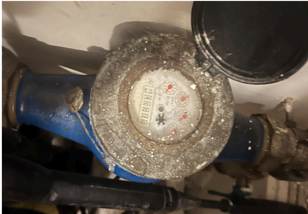
Figure 6: Veritas Water Meter
