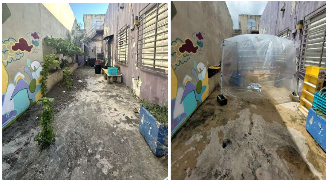
Figure 10: The alleyway next to the Gandul Community center before construction (left) and after hydroponic construction (right).
