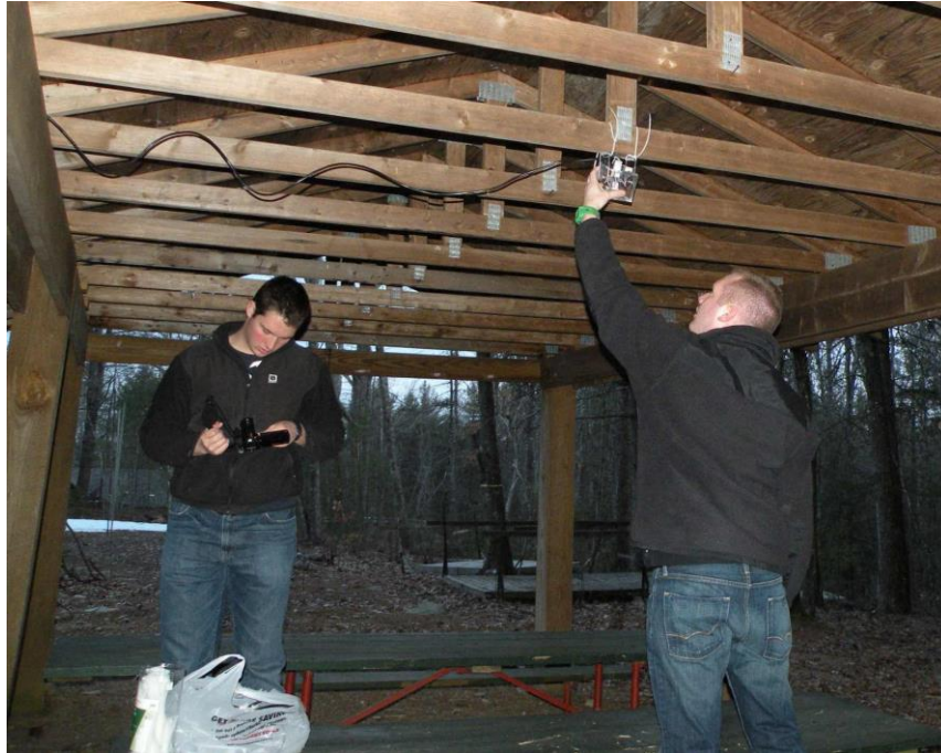
Figure 44: Light installation in pavilion
