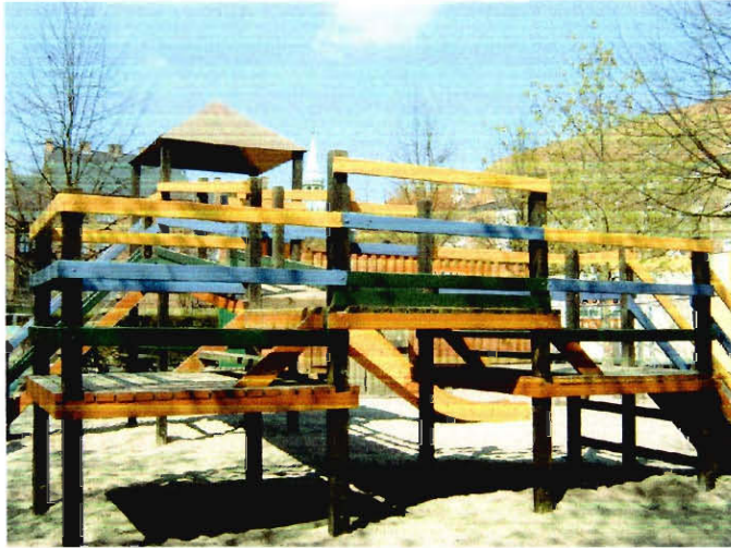
Fig. 4.17: Unsafe Barriers on Climbing Structure
