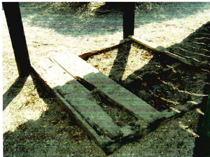
Fig. 4.13: Piece of Dangerous Wood
