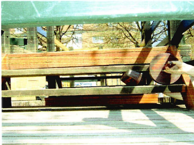
Fig. 4.15: Head Entrapment Test Failing on Stairs
