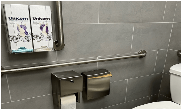
Figure 13: A Unicorn dispenser installed in a stall, right next to the toilet for easy access to menstrual products. (Unicorn, 2023).
