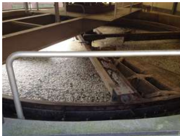
Figure 14: Gardner WWTF gravity thickener
