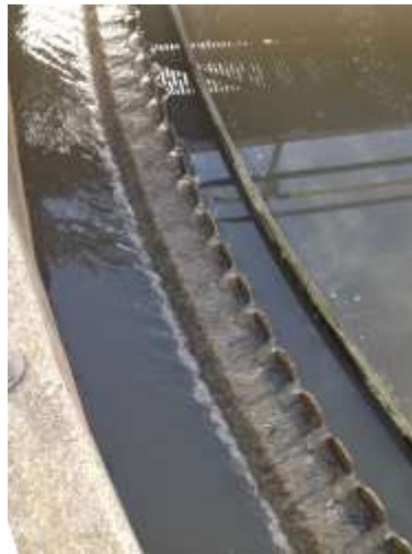
Figure 20: Location of primary clarifier sampling
