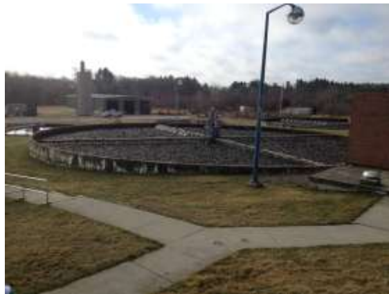
Figure 10: Trickling filters at the Gardner WWTF
