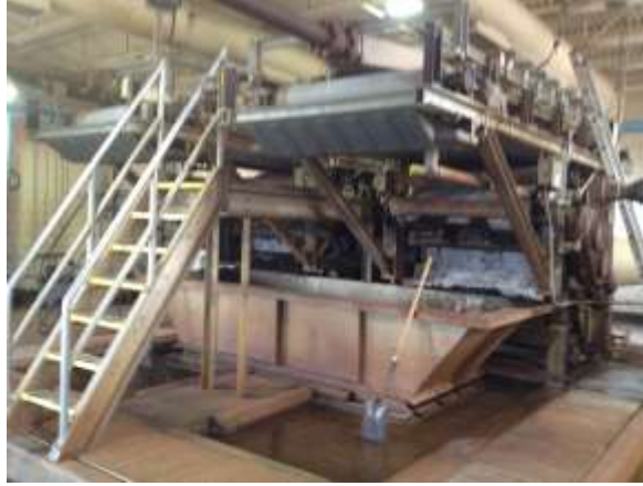
Figure 15: Belt press at the Gardner WWTF
