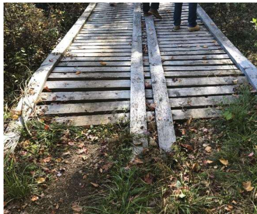
Figure 2: This wooden bridge on the existing path allows the road to continue through the wetlands on either side.
