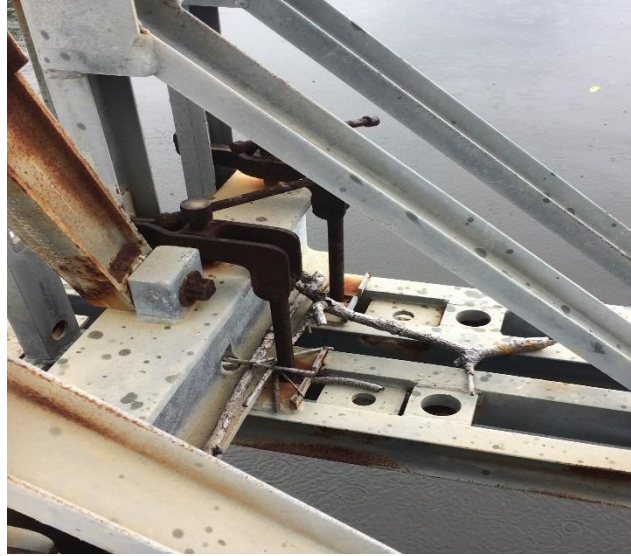
Figure 7. Bridge in Los Machos showing signs of corrosion and woody debris from flooding.
