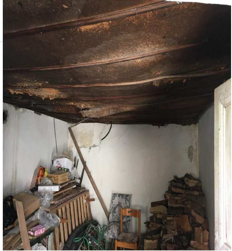
Figure 50 Example of a Very Bad Ceiling
