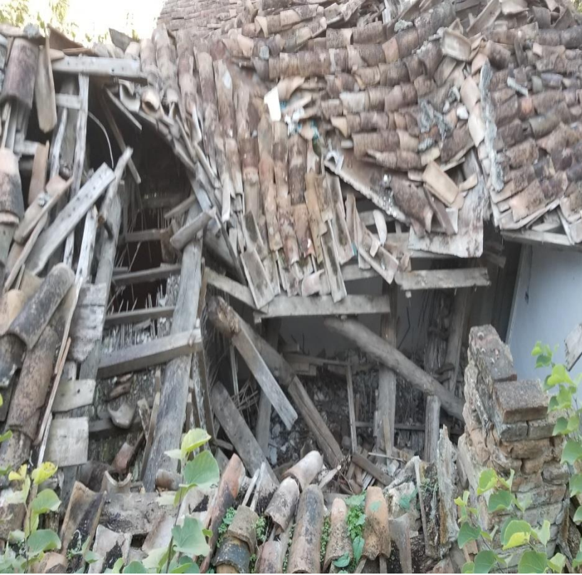
Figure 49 Example of Very Bad Roof
