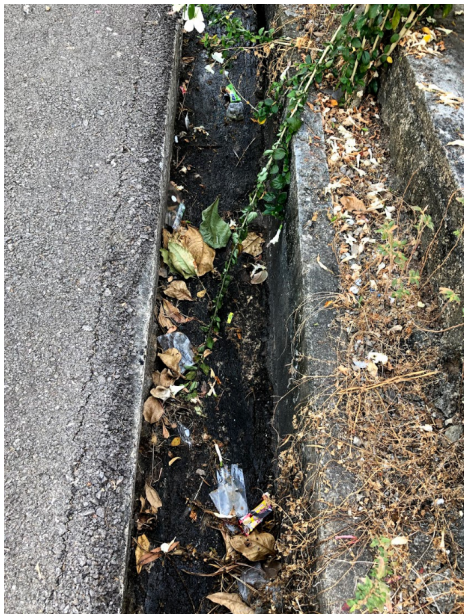
Pollution found in the sewer by the school
