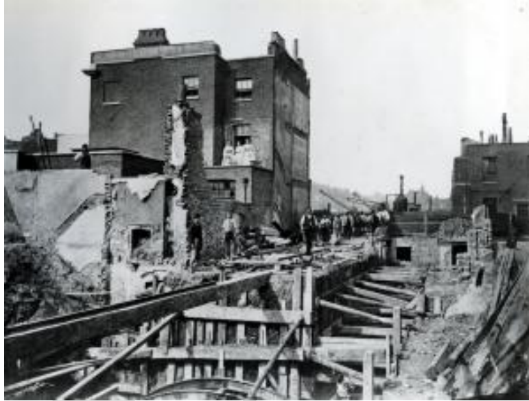
Completing tunnelling along Praed street, Paddington for the Metropolitan Railway's Kensington extension, c1866. Taken from the London Transport Museum's Online Collection (Reference: 1981/535)
