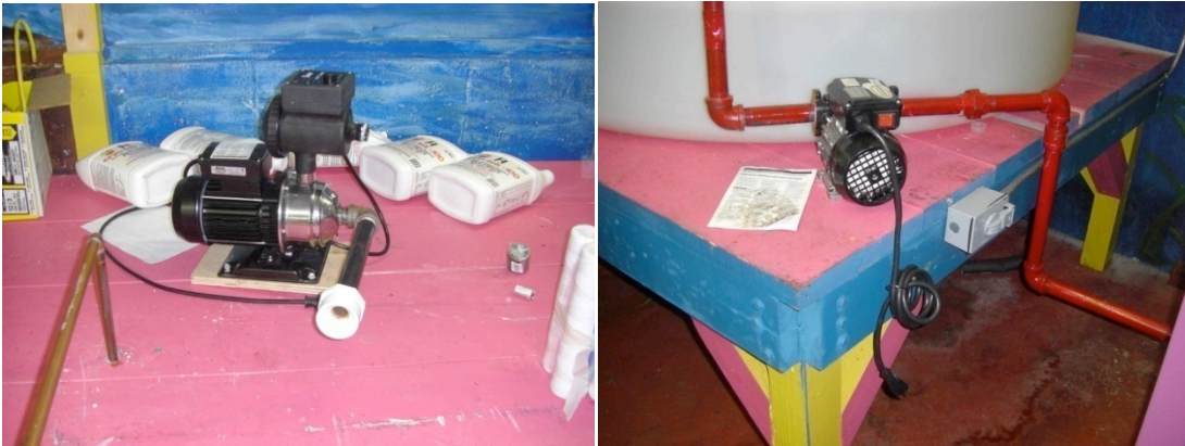
Figure 1: Small Storage tanks and pumps to move WVO, Hubbardston, MA
