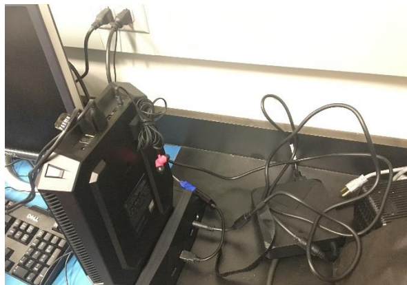
Figure 7.32 Power Connection From Outlet to Charging Base
