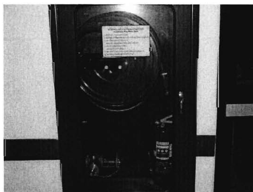
Figure 7: Fire Extinguisher and Automatic Hose Reel
