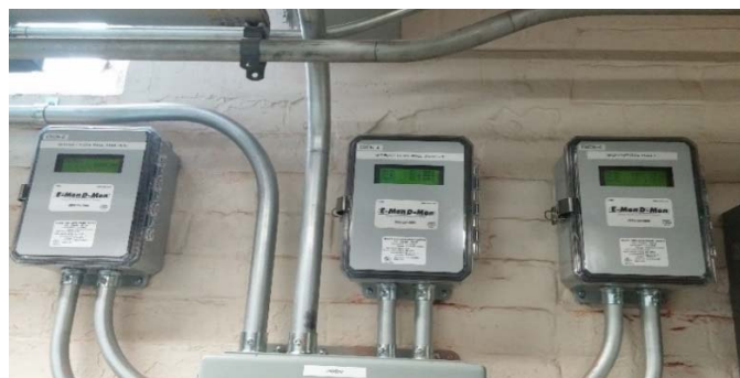
Figure 22 - E-mon Demon Smart Meters WPI Powerhouse
