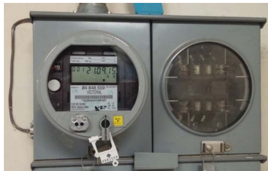
Figure 21 - WPI Powerhouse electrical sub-meter
