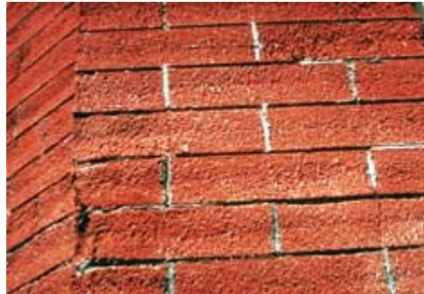
Historic brick damaged by sandblasting.
