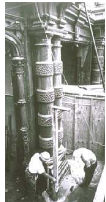
Missing cast-iron elements replaced with cast aluminum.
