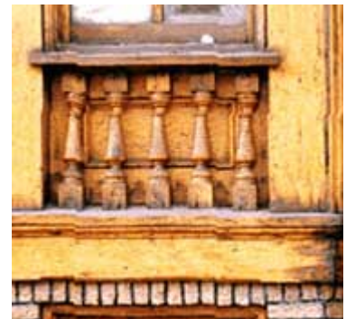
Wood features inappropriately stripped of traditional painted finish.
