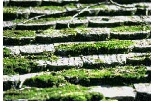
Moss on wood shingles indicative of damaging moisture retention.
