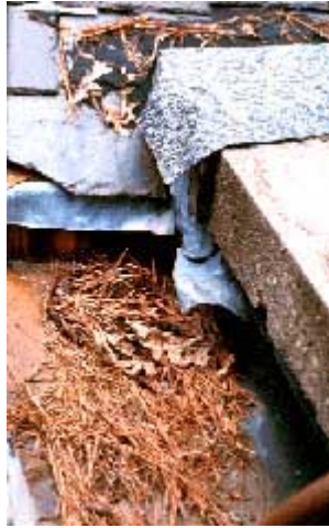
Clogged gutter leading to corrosion.
