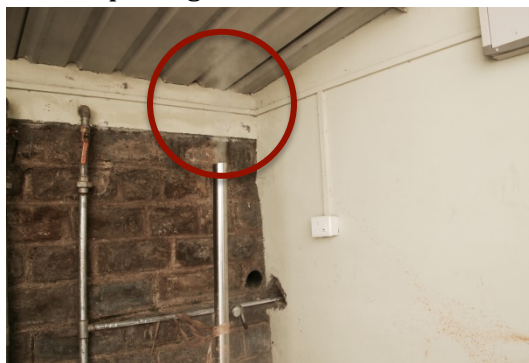
Figure 11. Smoke escaping from top back pipe during testing (Zhang, 2016)
