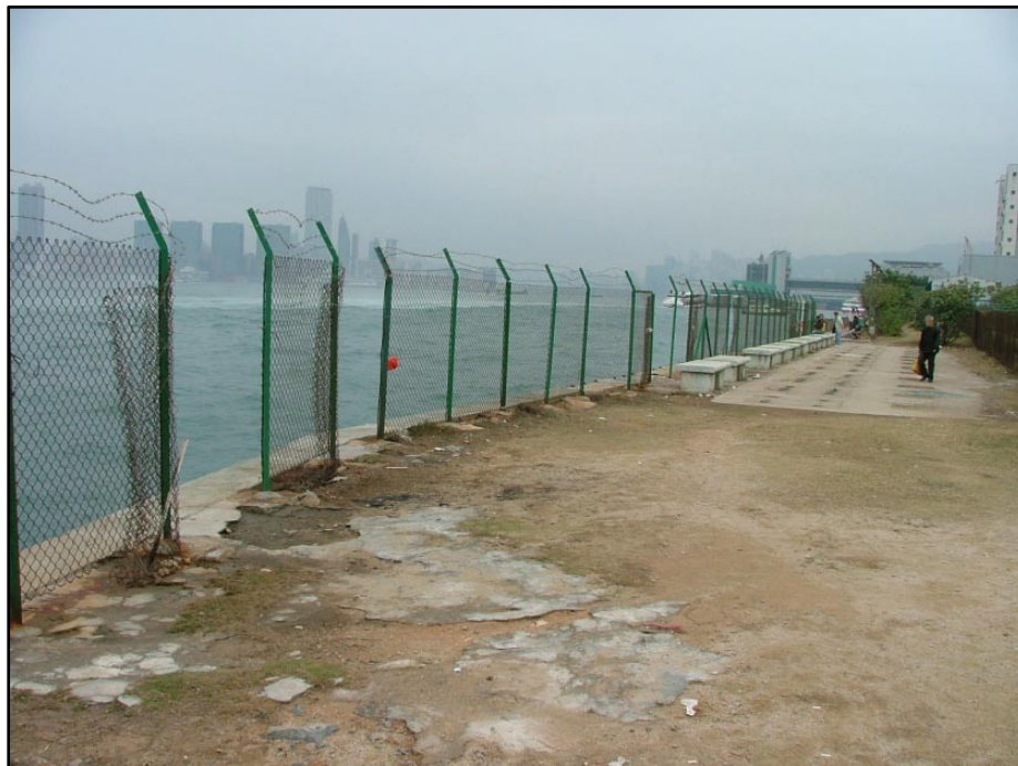
Figure 5.15: Dilapidated walkway and fencing at west end of Sheung Wan
