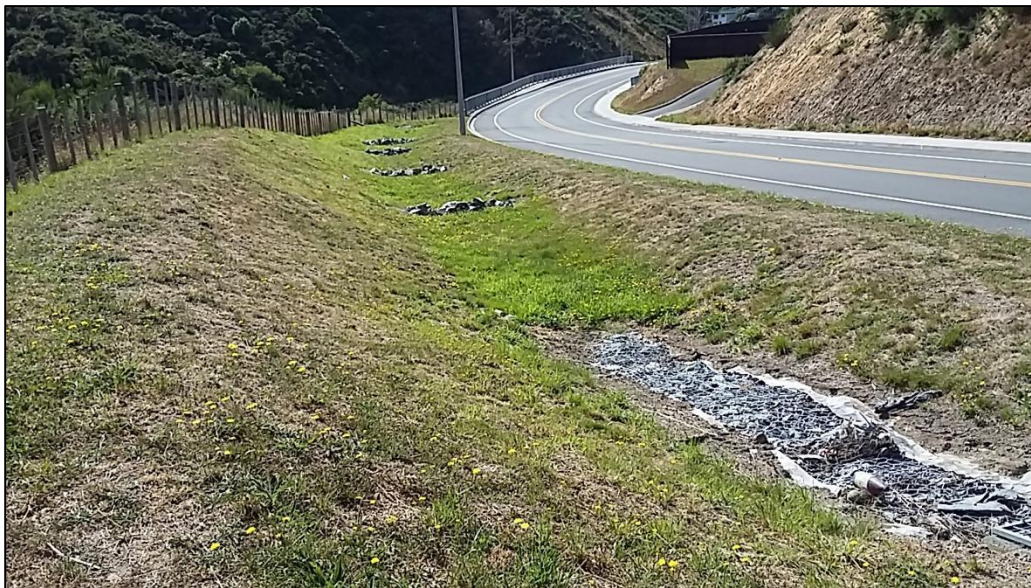
Figure 8: Swale in Porirua
