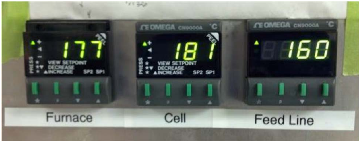
Figure 58 Temperature control boxes
