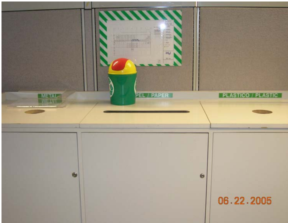
Figure 5: Disposal Containers in the Office Area at Intel
