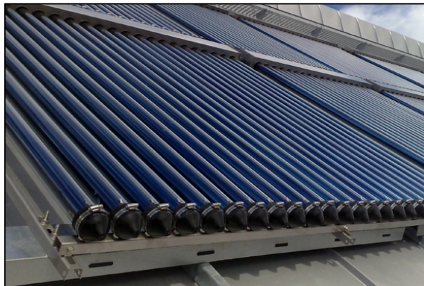
Figure 14 - A thermal solar panel installation [19].
