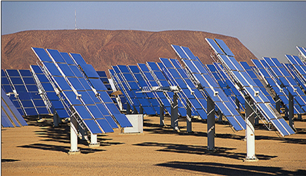
Figure 17 - Multiple PV panels mounted on the ground [22]
