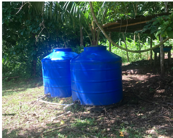
Figure 16: Water storage tanks located near Cabimos (Konsko, 2017)
