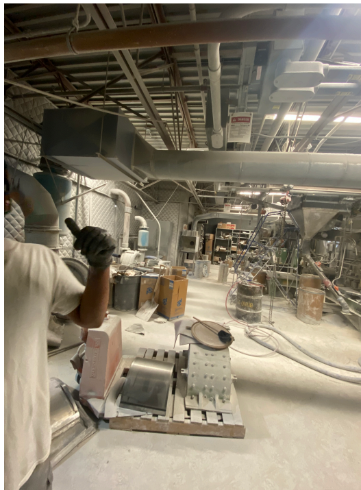
Figure (16) - Walkway Clutter in Workspace
