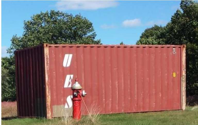
Figure 6: Fire hydrant on Mixer property from team site visit.
