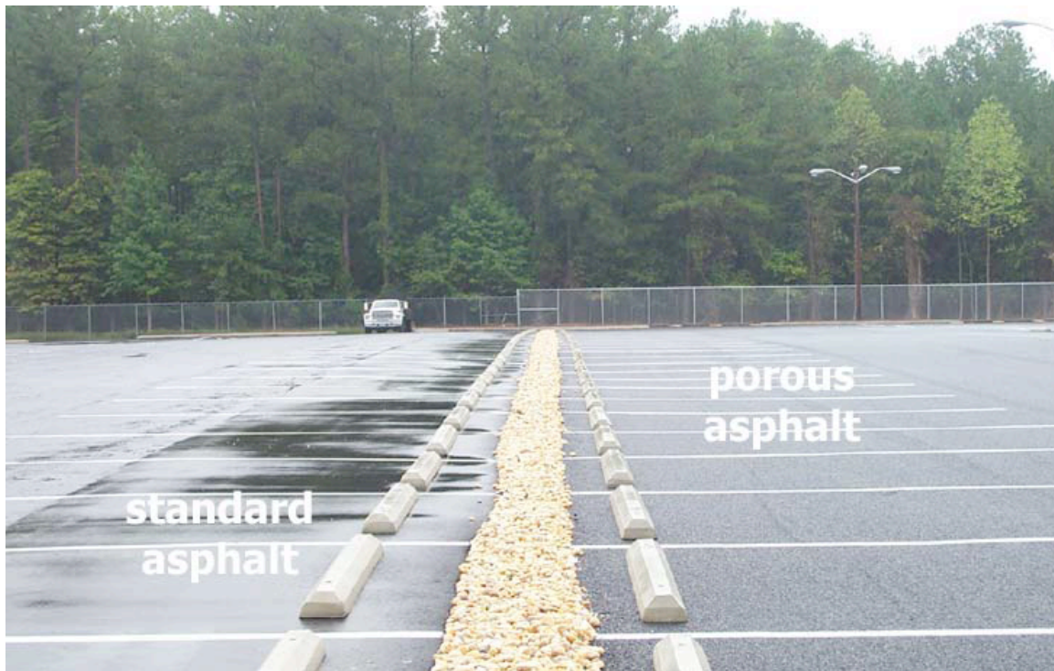
Figure 13: Parking Lot With Both Typical and Pervious Pavements After Rain 32
