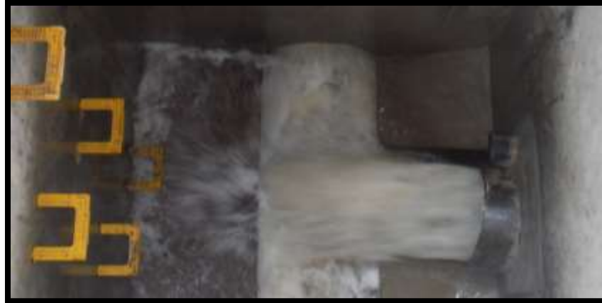
FIGURE 8: TREATED WATER LEAVING THE UJAMS RECLAMATION PLANT
