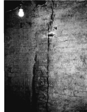
Figure 22- Crack and Strain Gage
