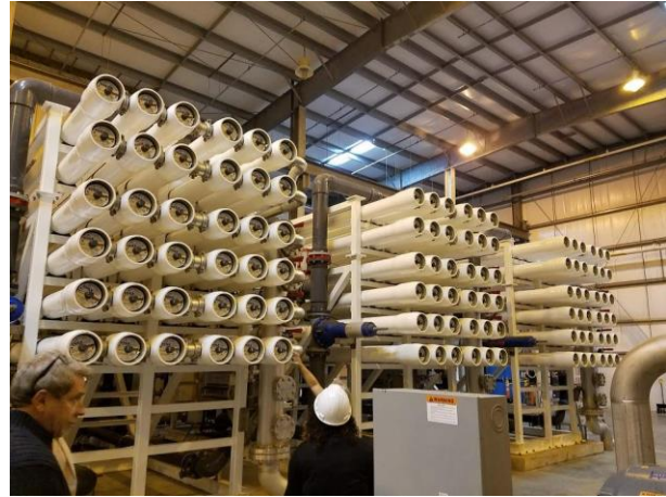
Figure 2: Reverse osmosis trains in TRDF
