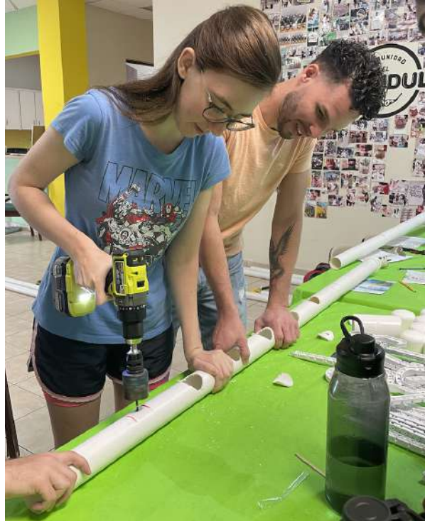
Figure 26: WPI Student team and local partners drilling holes into the PVC water troughs for the Hydroponic Garden
