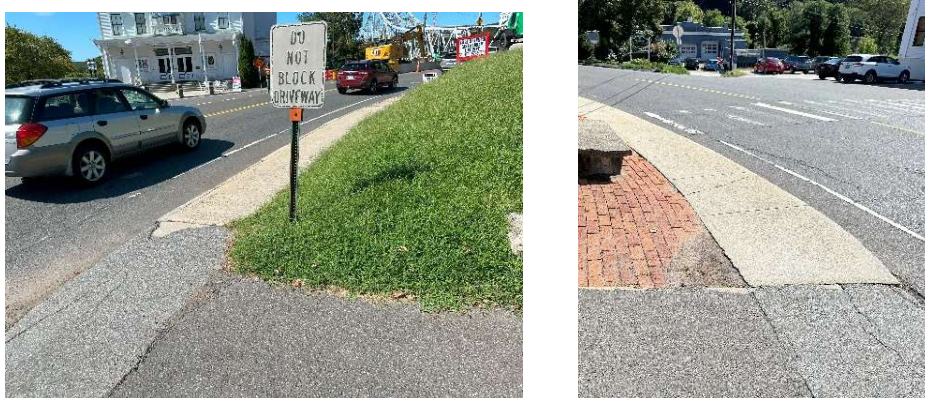
Figure 4a (left) and Figure 4b (right). Narrow sidewalk on southbound lane of Route 82 in the EHVD (Swann, September 14, 2023).
