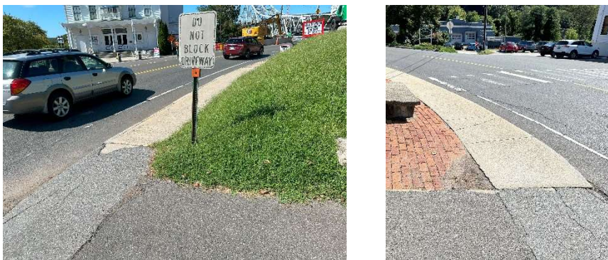
Figure 4a (left) and Figure 4b (right). Narrow sidewalk on southbound lane of Route 82 in the EHVD (Swann, September 14, 2023).
