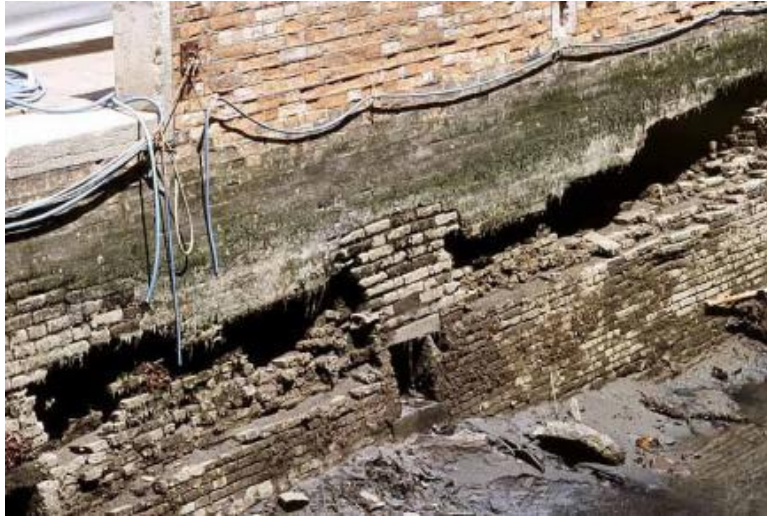
Figure 12: A damaged canal wall 33
