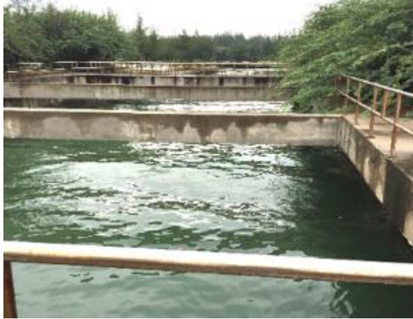
Figure 7: Inside feature that allows seawater to enter the forest through the jetty
