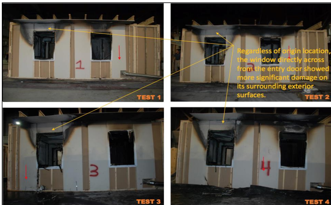
Figure 43: Exterior Window Wall Damages
