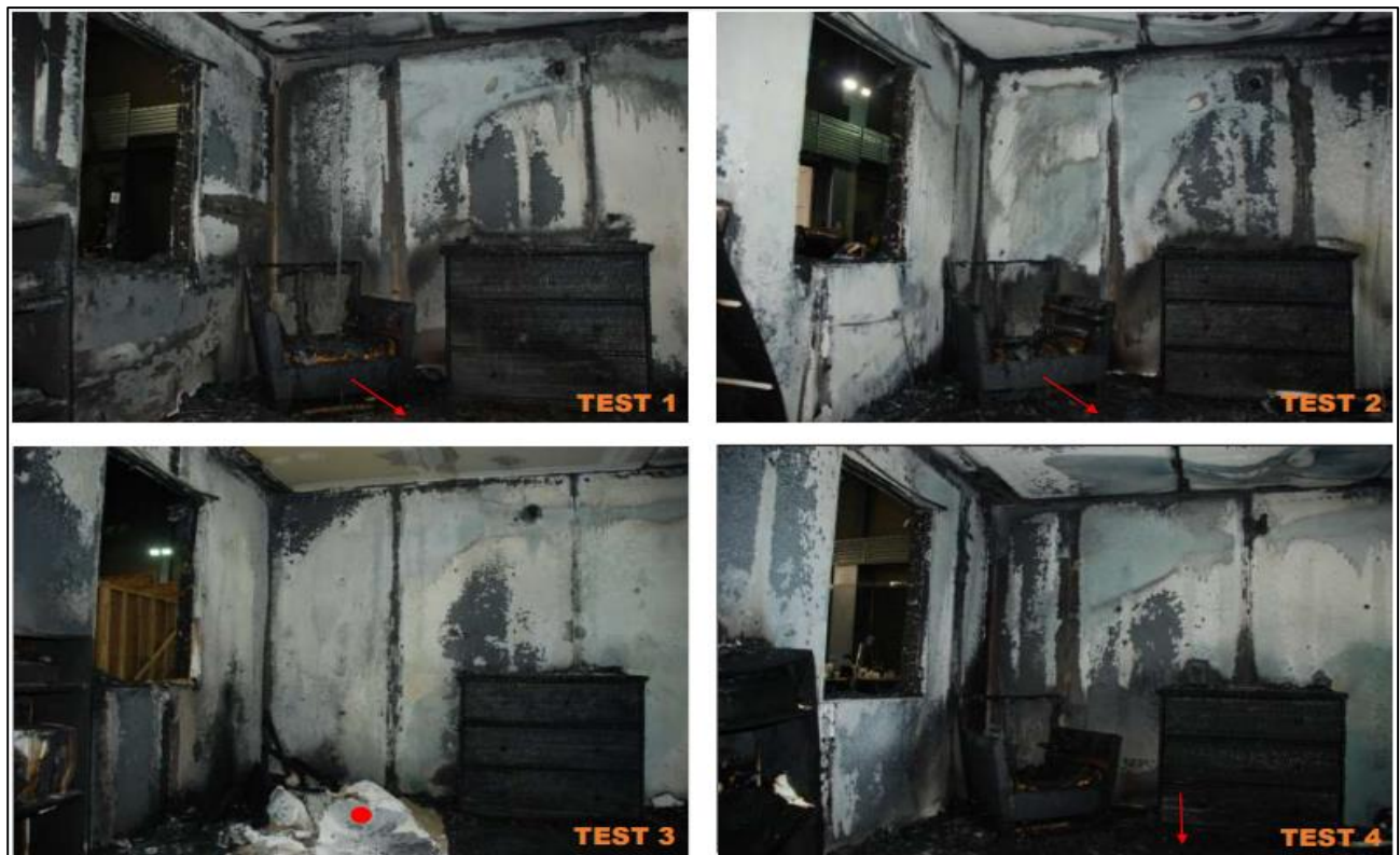
Figure 45: Quadrant 2 Corner Wall Damages
