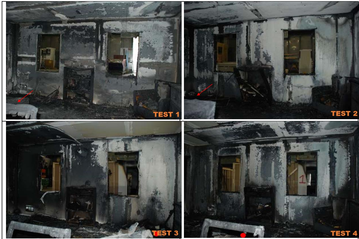
Figure 44: Interior Window Wall Damages
