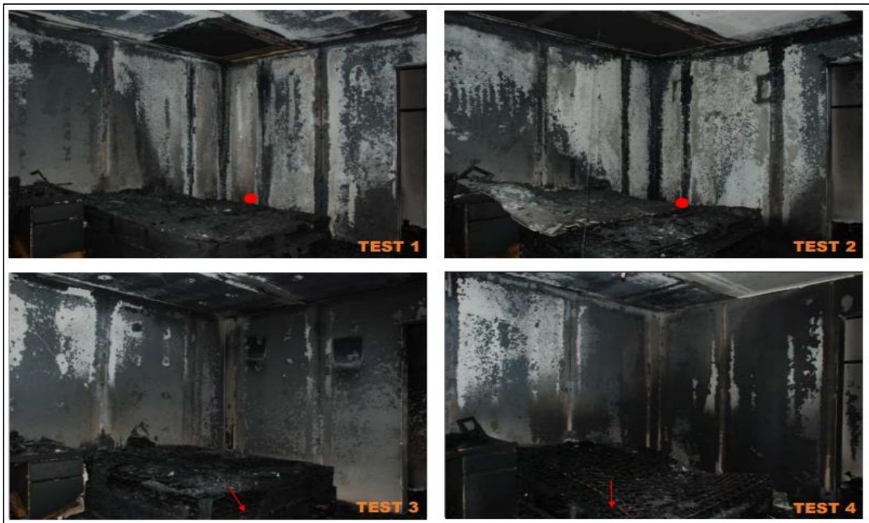
Figure 47: Quadrant 3 Corner Wall Damages
