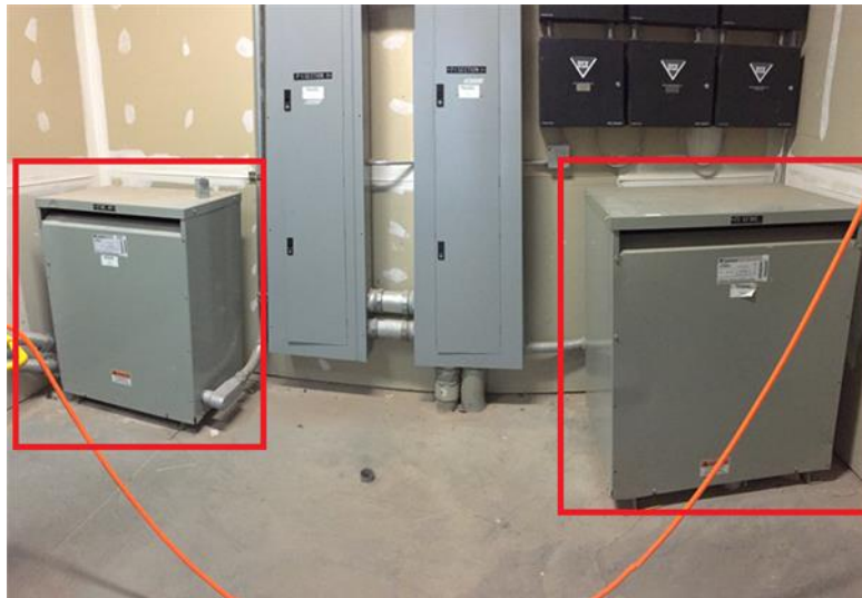
Figure 12: Transformers in the AB
