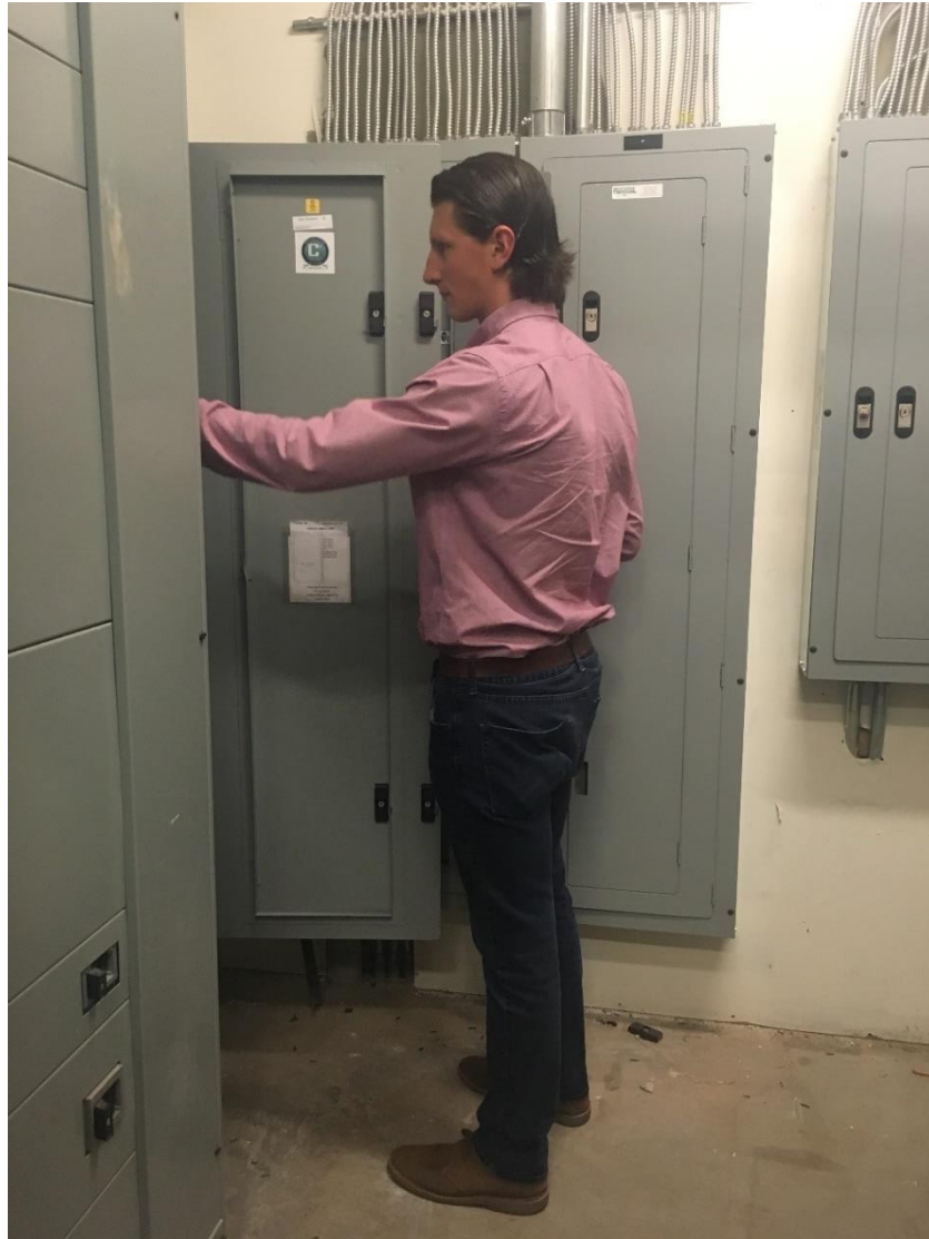
Figure 16: Collecting information on the electrical panels in the AB
