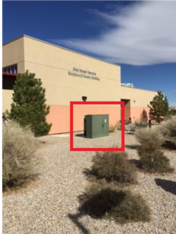
Figure 15: The Foundry's transformer
