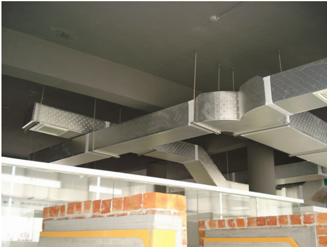
Figure 4.6.1(Air Duct for Central Air Conditioner)
