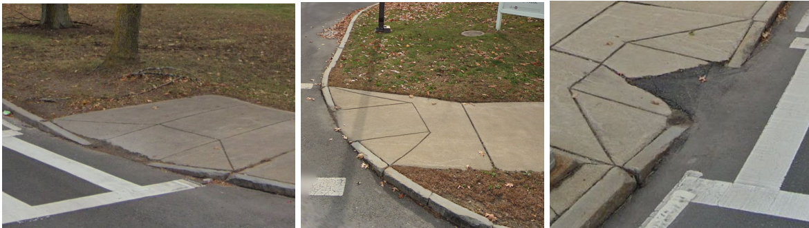
Figure 14: Non-compliant wheelchair ramps at intersection of Market Street and Broad Street (left) and along the Lynnway (mid) and at the rotary (right) (Google Earth, 2020)
