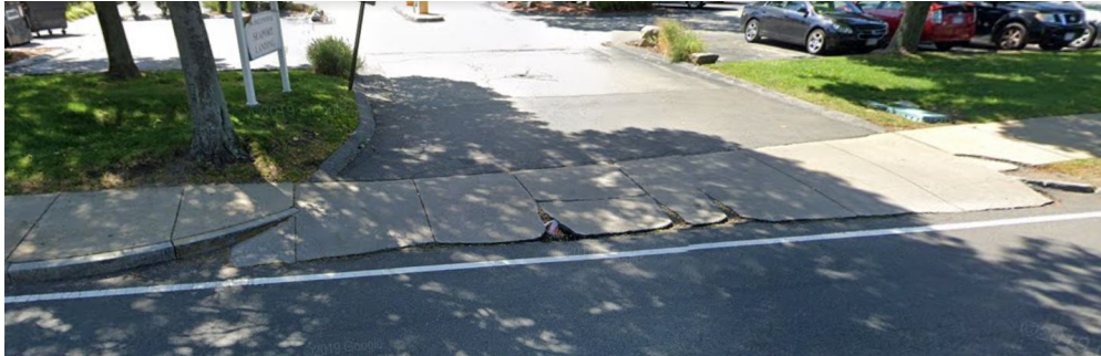
Figure 16: Dangerous sidewalk at a driveway at 150-154 Lynnway (Google Earth, 2020)
