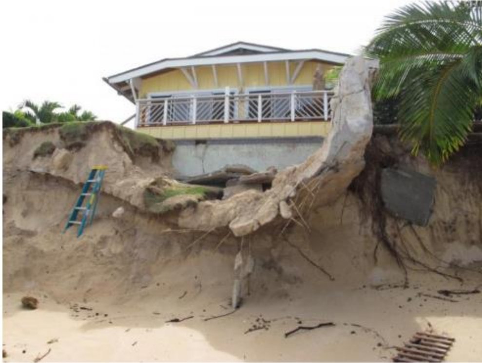
Figure 11. Property damage caused by SLR and beach erosion (NOAA, 2017)
