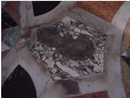
Figure 26: An example of floor replacement found in the Santa Maria Della Salute
