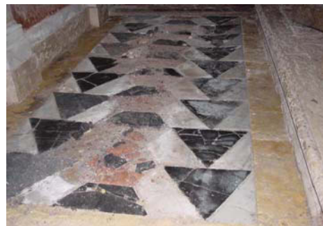
Figure 3: Severe wearing found in the San Marcilliano
