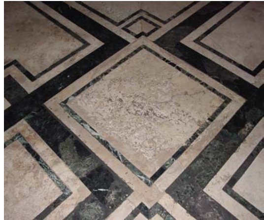
Figure 23: Pitting of the floor seen in the Santa Maria Assunta dei Gesuiti .
