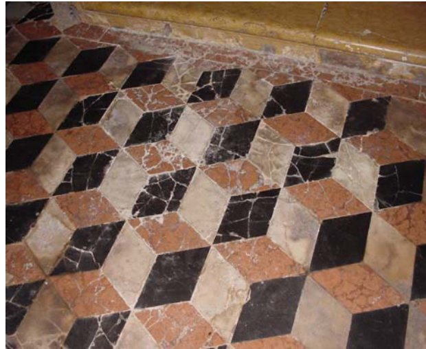
Figure 22: An example of cracks seen in the Santa Maria Assunta dei Gesuiti .
