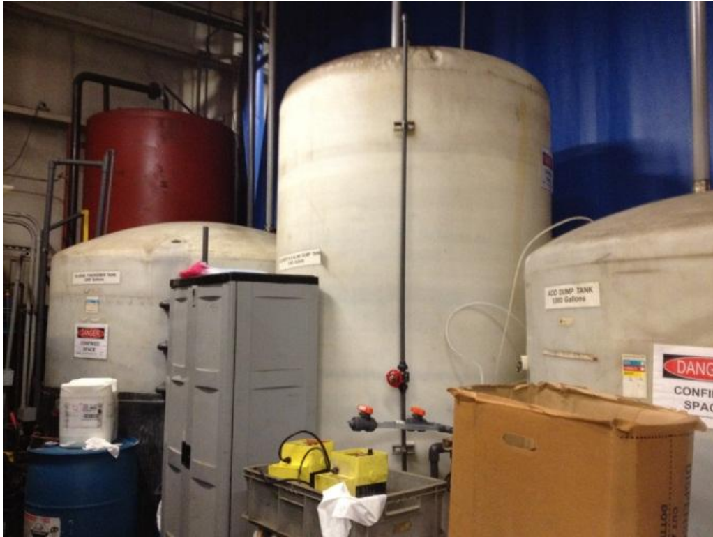
Figure 5: Wastewater Line Lift Stations
