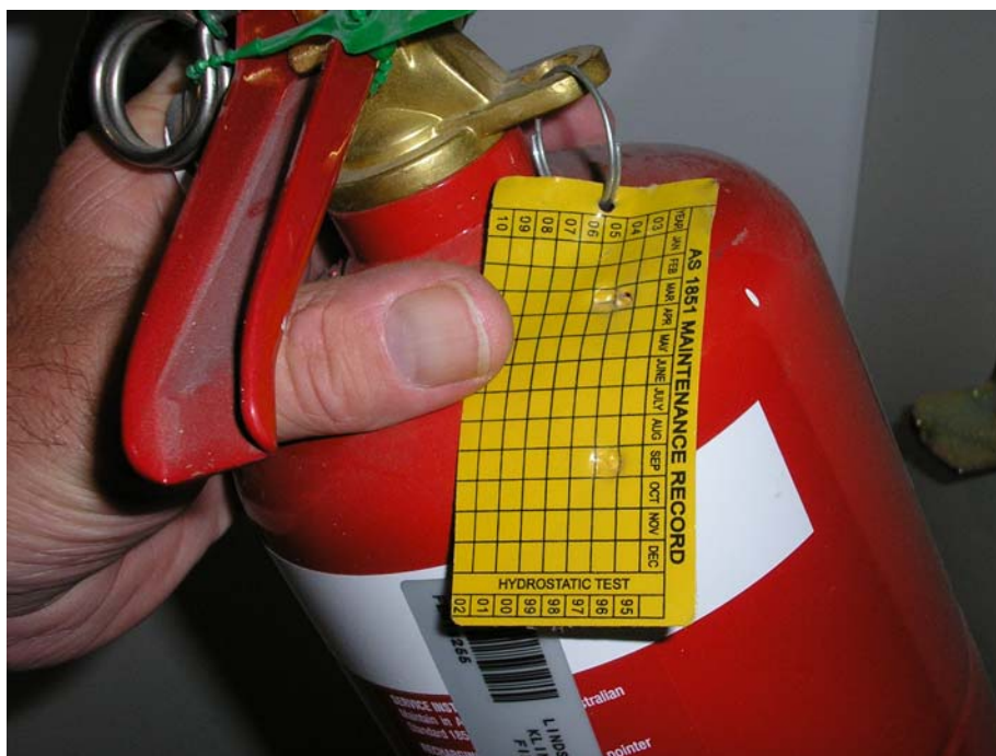
Figure 12-1: Overdue Maintenance on Fire Extinguishers in Building B
