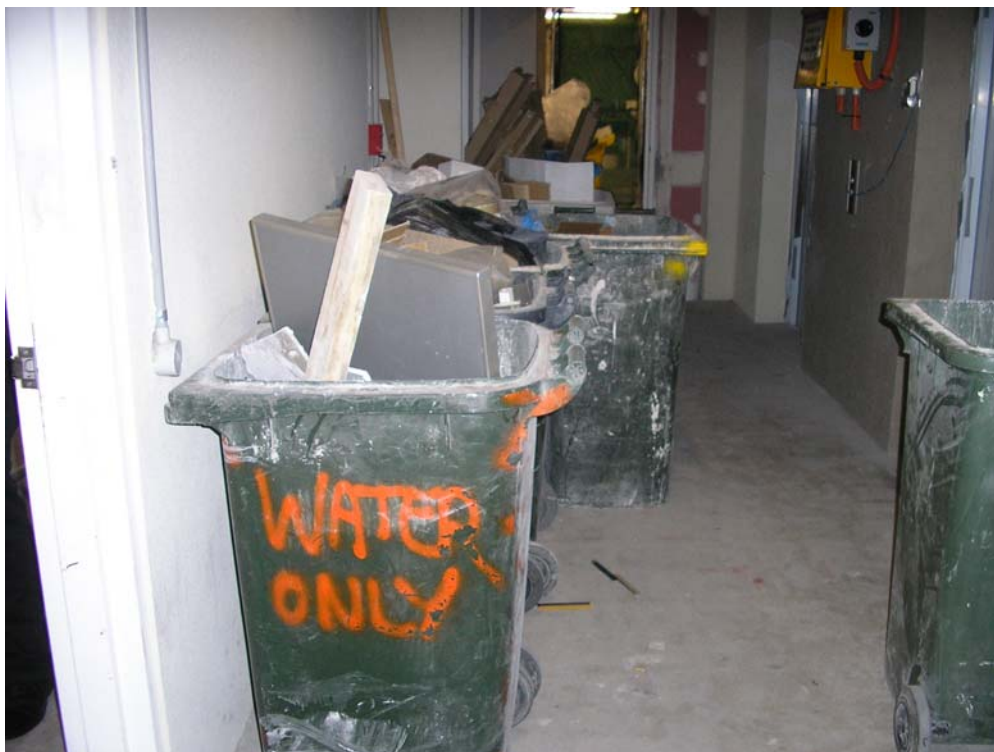
Figure 12-2: Rubbish in First Floor Lift Lobby of Building C
