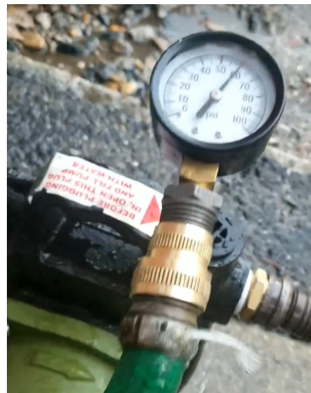
Figure 22: Pressure gauge attached directly to hose outlet
