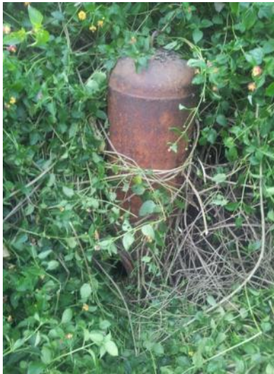
Figure 21: Unused Water Pump in Neri
