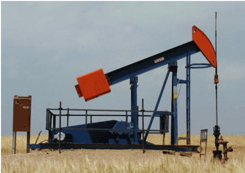
Figure 22 - Oil Pump Jack
