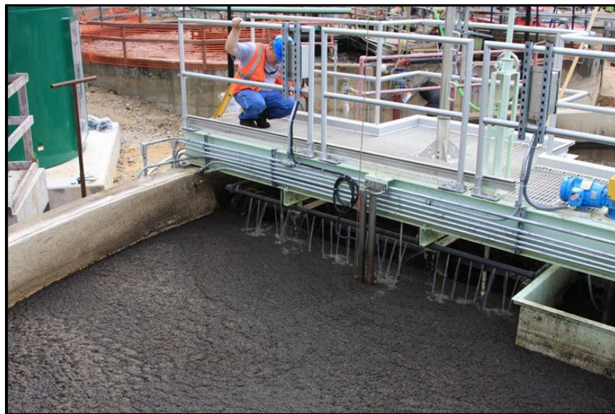
Figure 2.8: Foam Surface Wasting, PTU #1
