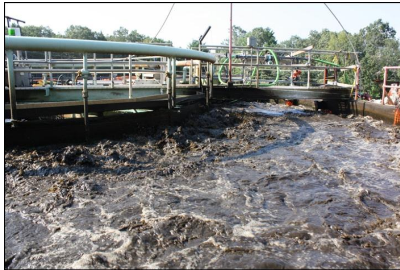
Figure 2.5: PTU #2 Aeration Tank (Pre-Upgrade)
