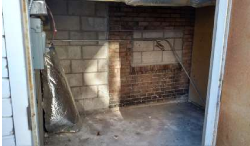
Figure 4-2: The inside of the shed behind the Sustainability Hub where the cistern could potentially go.
