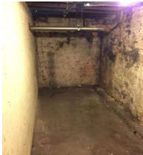
Figure 4-3: Location in the basement of the Sustainability Hub where the cistern could be located
