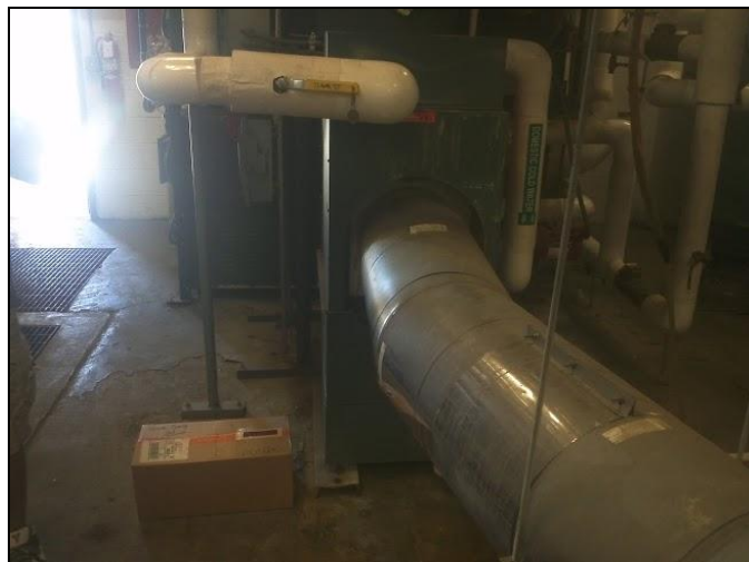
Figure 3.1 b: Picture of the Raypak Units (Fay, 2015)
