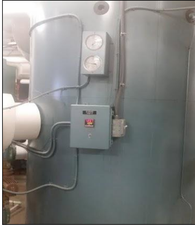
Figure 3.1 c: Picture of the Storage Tanks (Fay, 2015)
