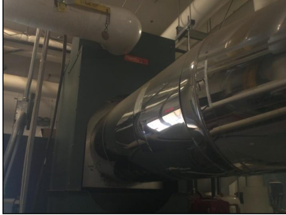
Figure 2.6 a: Picture of Raypak Units in Worcester County Jail (Fay, 2015)
