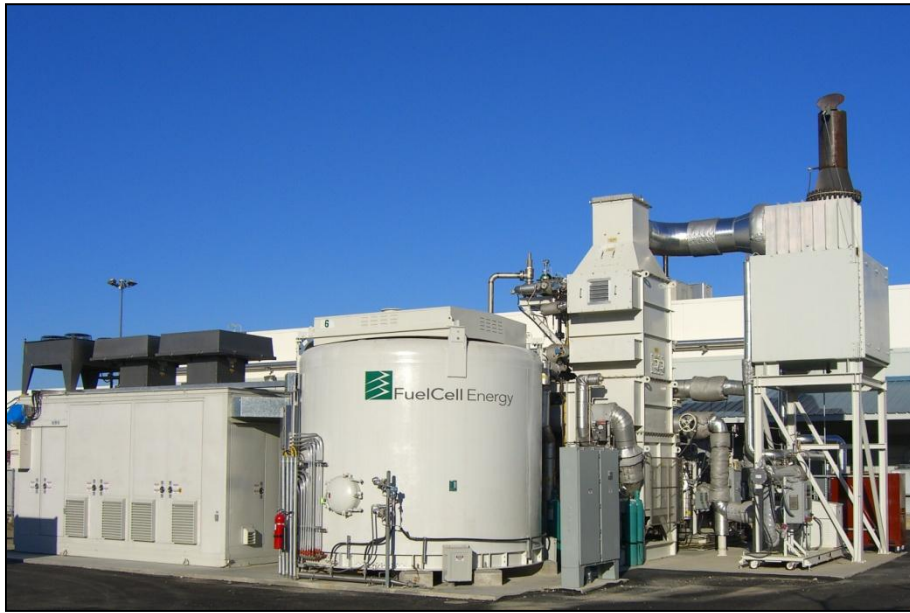
Figure 2.2 g: Picture of Fuel Cell CHP unit implemented at Santa Rita Jail (Alameda County, 2013)
