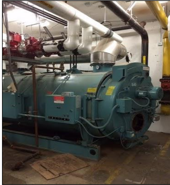
Figure 3.1 a: Picture of the Boiler from the Worcester County Jail (Fay, 2015)
