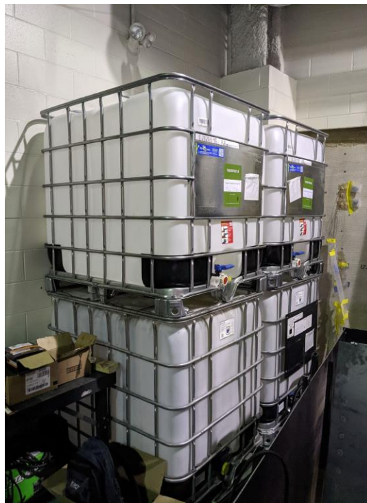
Figure 10: Water Storage Totes
