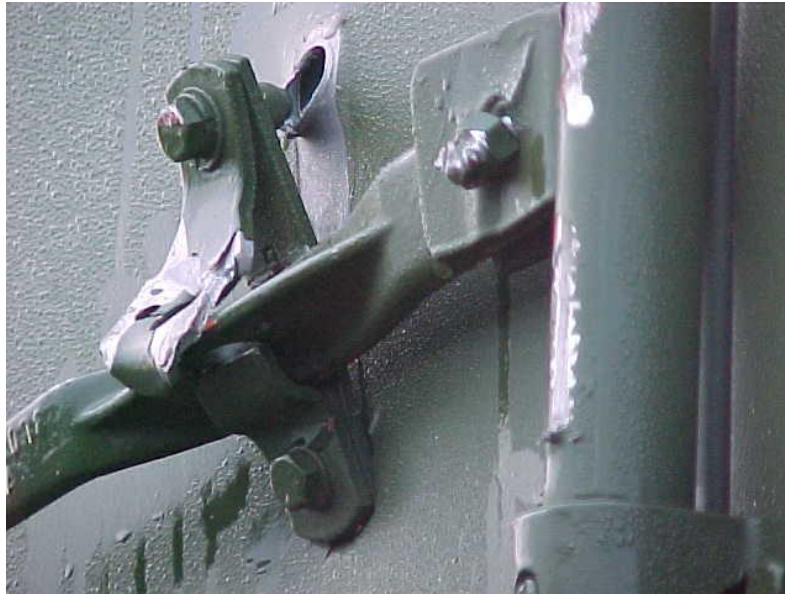
Figure 6: Failure of Exterior Connections [A.1]
